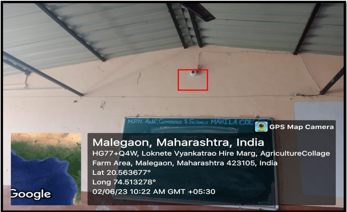
CCTV in Seminar Hall
